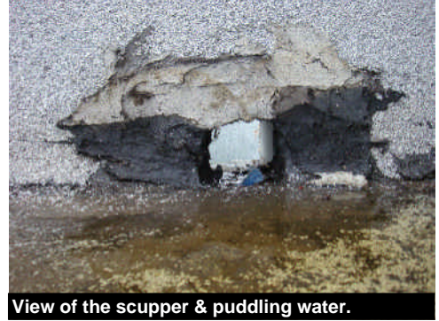
View of the scupper & puddling water.
