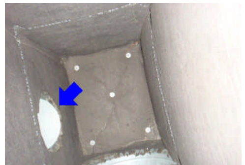
Damper at the plenum, controlled from duct
