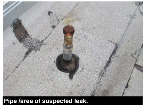
Pipe /area of suspected leak.
