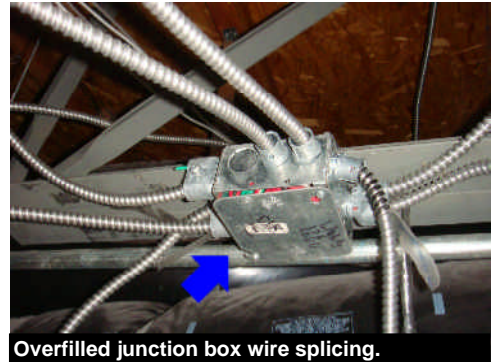
Overfilled junction box wire splicing.
