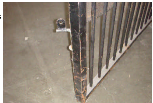
Gate is bent /damaged at bottom.
