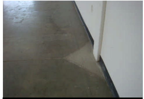
Grind the bolts down to prevent tripping.
