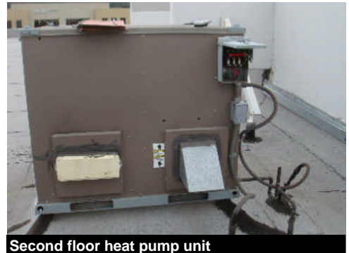
Second floor heat pump unit
