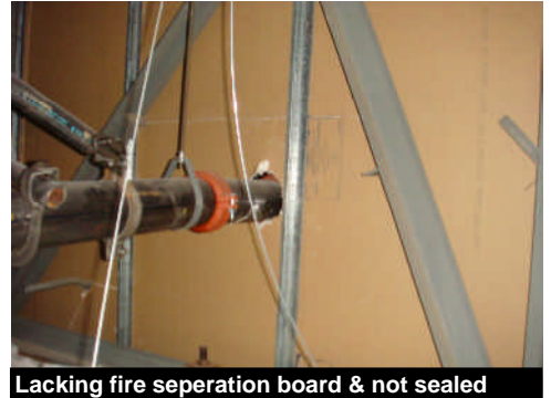
Lacking fire seperation board & not sealed
