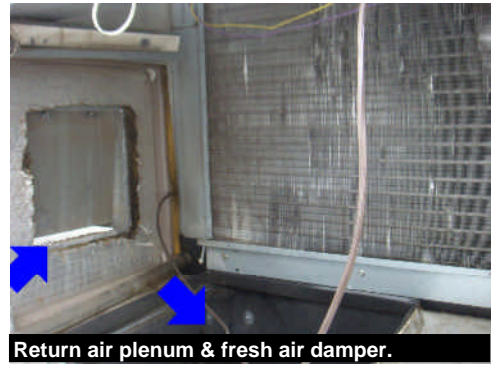
Return air plenum & fresh air damper.
