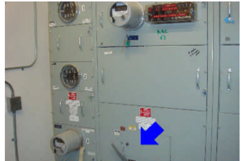
Main disconnect switch at main cabinet.
