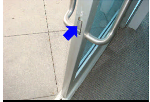
Door pin only latched by pushing up.
