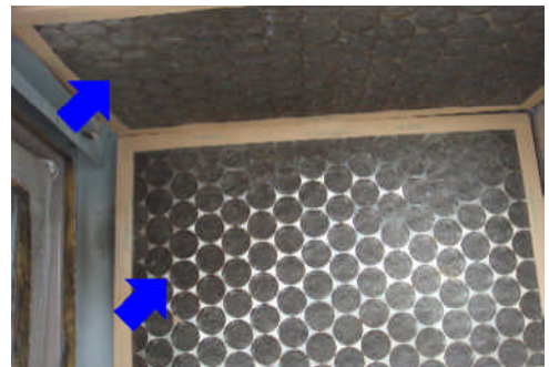
Cheap filters in the units.
