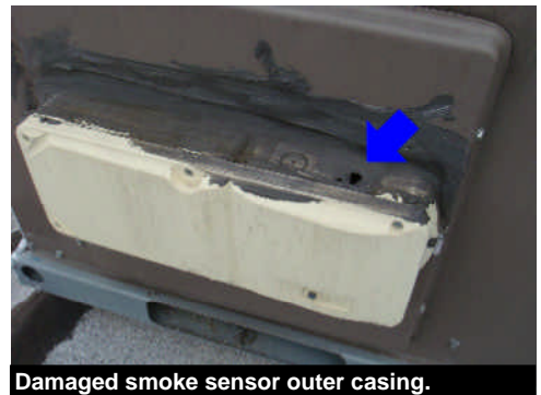
Damaged smoke sensor outer casing.
