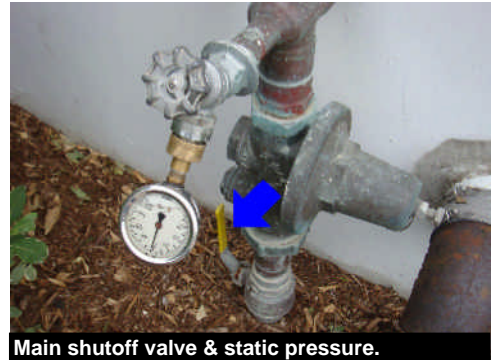
Main shutoff valve & static pressure.
