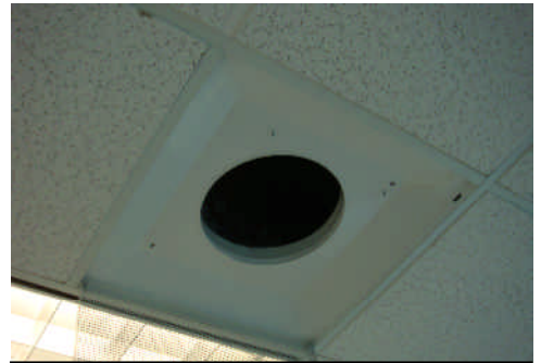
View of a return air duct /grill.
