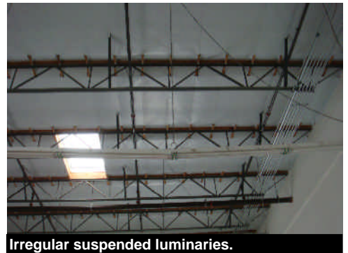
Irregular suspended luminaries.
