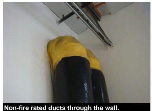
Non-fire rated ducts through the wall.
