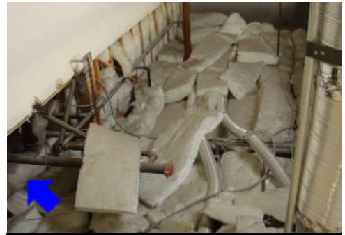
No fire separation wall /ceiling.
